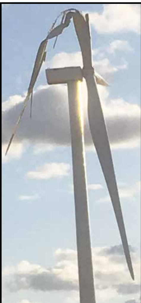
(Photo courtesy Mark Casey) A blade of a turbine on 861 Road has deteriorated and bent over. NextEra hypothesizes that the blade was defective.
